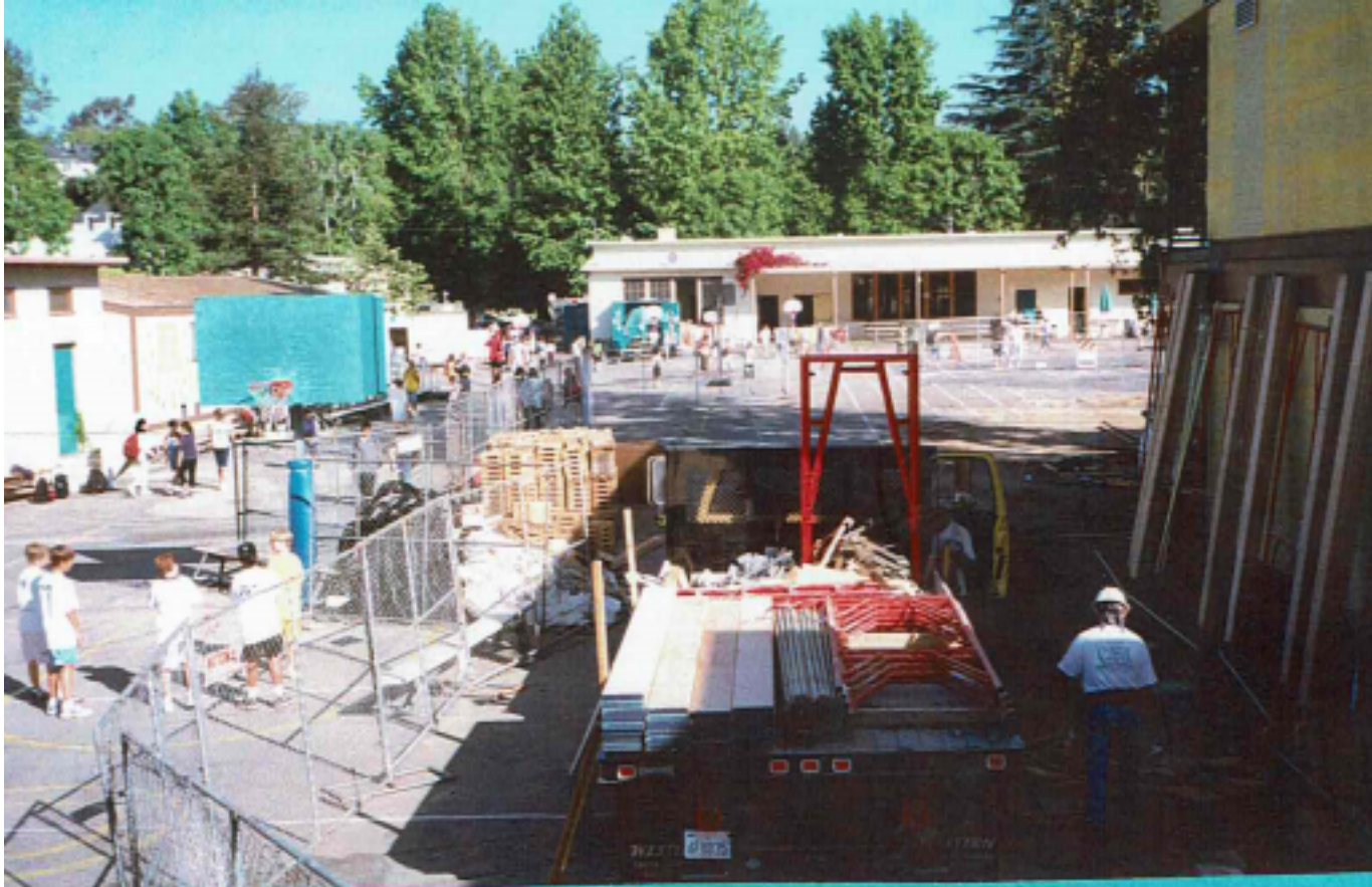
The view of construction from the library building, with your back to Woodruff looking towards Loring. Relocated bungalows on the left.
